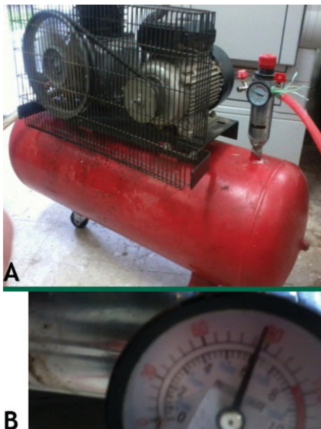
Fig. 1 Photograph of the air-drying pump (compressor).
